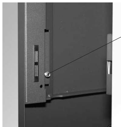
Fig. 24 Checking the setting of the door safety switch
