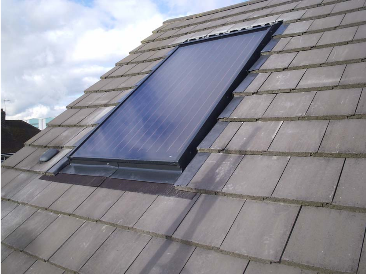
Baxi in-roof solar panel.JPG
